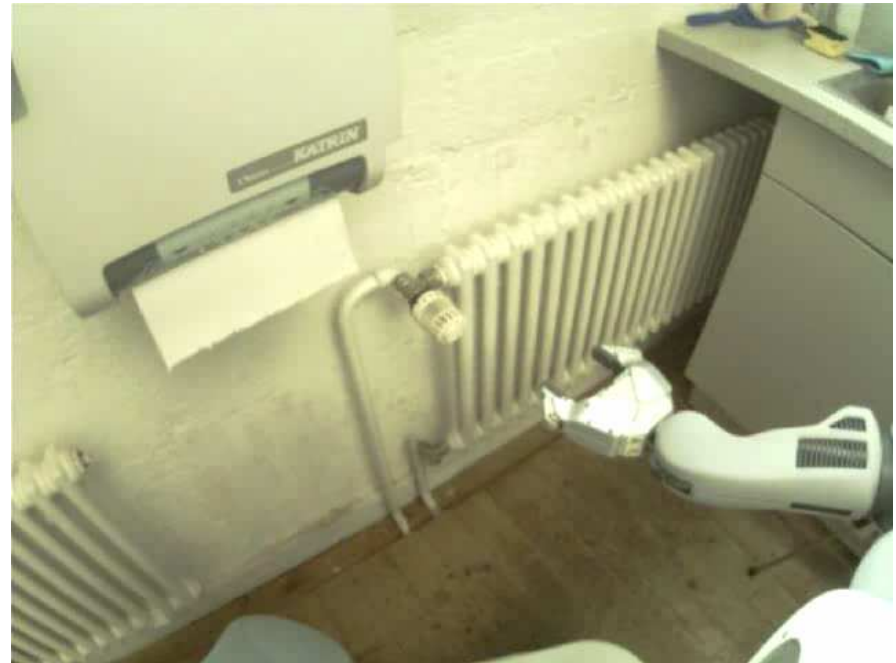
valve of a radiator
